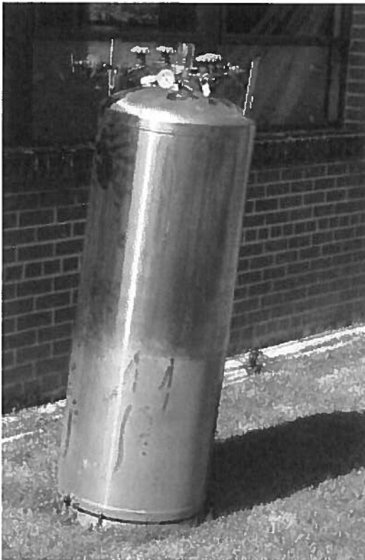
Figure 23. This liquid oxygen cylinder is not secured and appears like it could topple over very easily.
