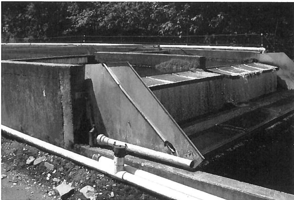
Figure 12. The white pipes in the foreground are part of a centralized vacuum system used to
