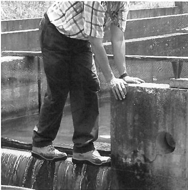
Figure 16. Walking on the raceway spillway is risky.
